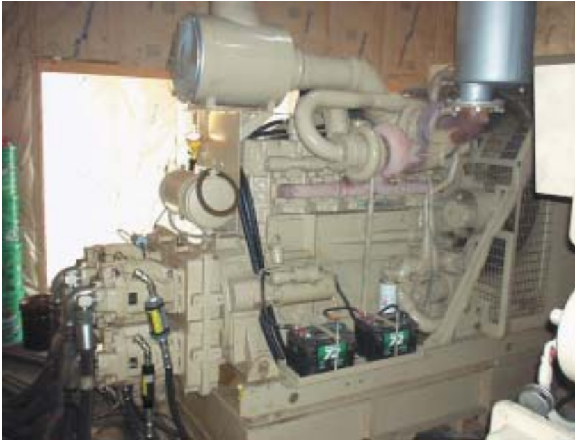
Each of two hydraulic power units is driven by a diesel engine coupled to a four-station pump drive box.
